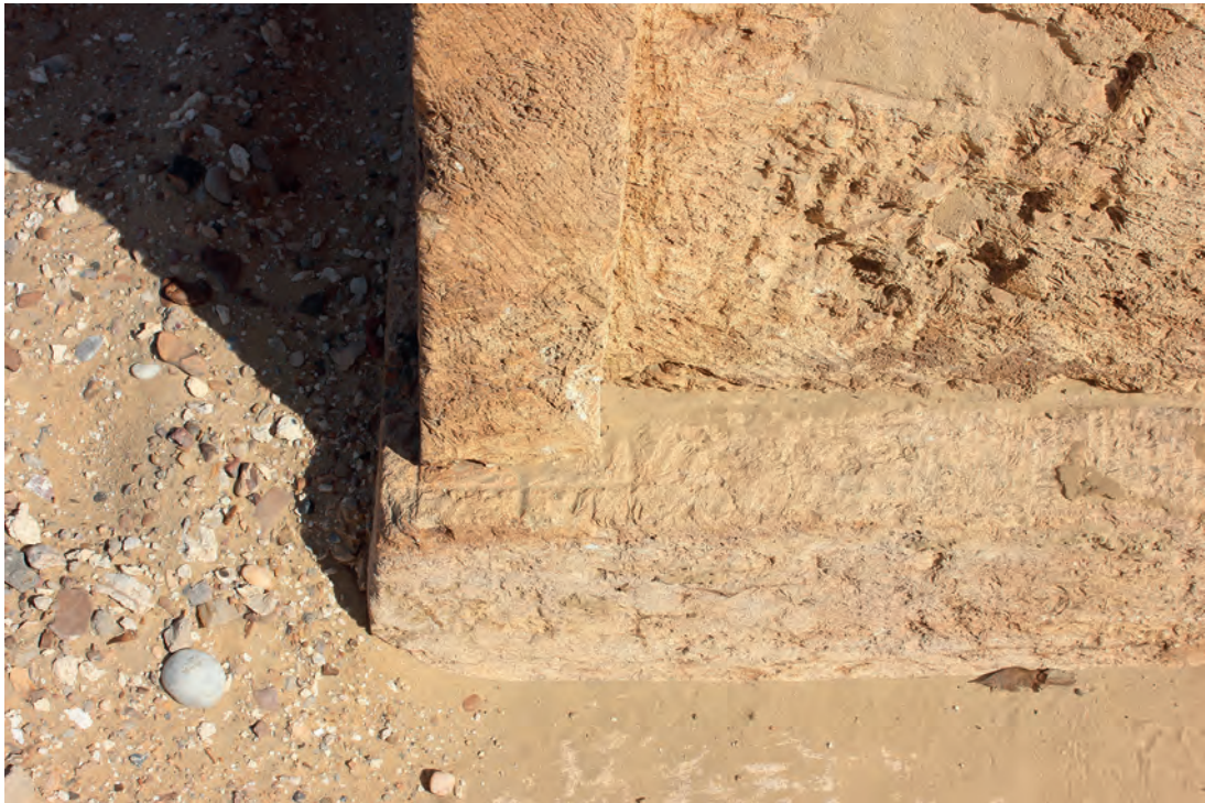
Fig. 6: Incision on top of the euthynteria indicating the future position of the round bar of the southwestern corner of the naos; 2015
